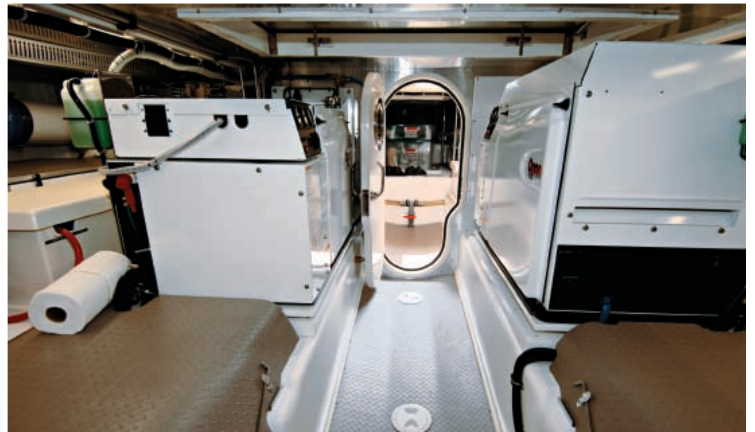
Top: Looking forward at the starboard engine installation. Notice the polished stainless-steel mirror that reflects the outboard side of the engine, as well as the large fiberglass cover over the otherwise exposed running gear and Aquadrive thrust bearing. Above: Looking aft in the engine room shows a clean machinery space, with twin Onan generators, relatively wide access door into the lazarette, and increased headroom in the newer boats.
