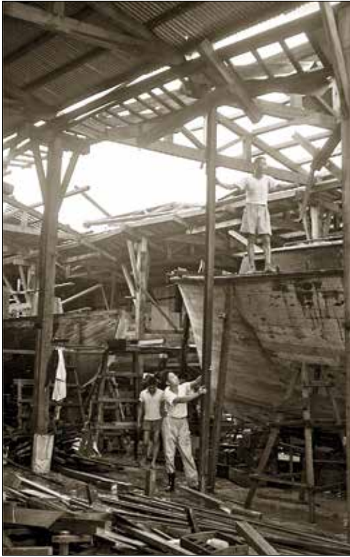
Crews inspect and shore up the American Marine boatbuilding facility in Junk Bay, Hong Kong, in the aftermath of Super Typhoon Wanda, which hit September 1, 1962, just three months after Fleming began overseeing engineering for the yard.
