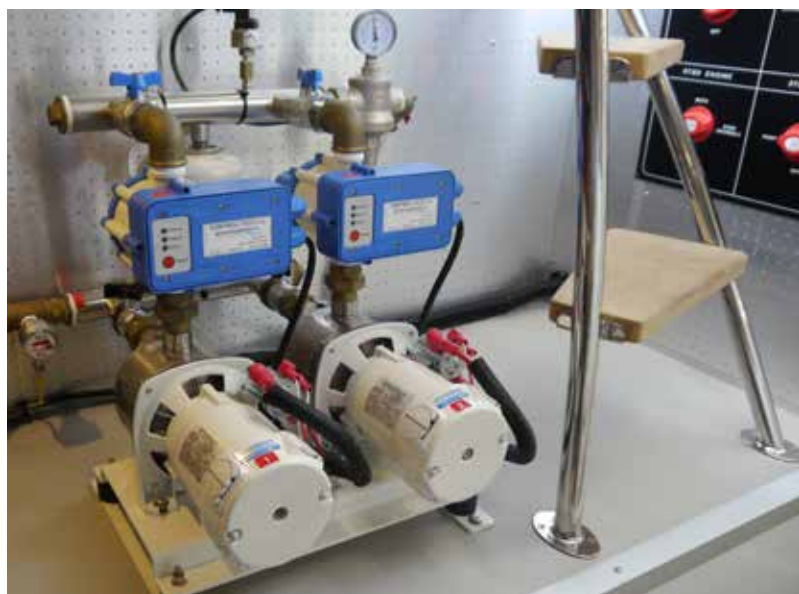
Dual fresh water pumps
