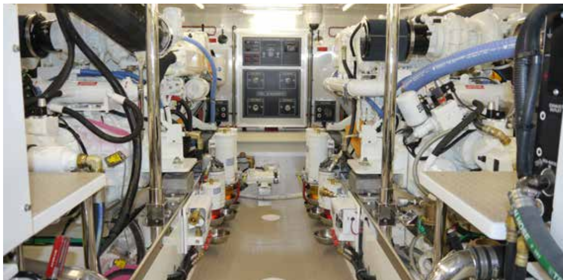
Fleming 65 engine room
