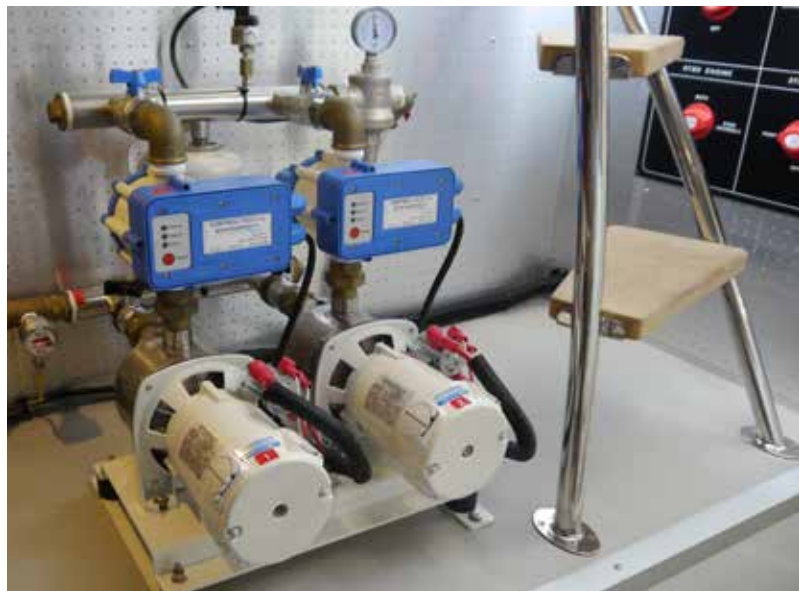
Dual fresh water pumps
